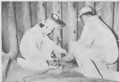
Skilled welders here pause briefly before continuing their task of fitting back the tubes in the KHAR furnace.
